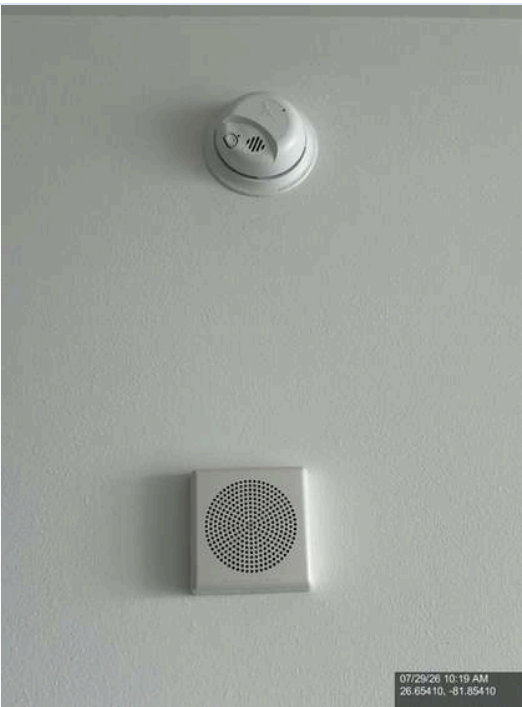
Photo 11 - Mechanical & Systems - Smoke and carbon monoxide detectors
