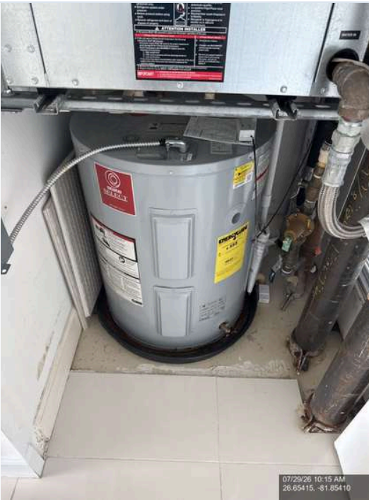
Photo 9 - Mechanical & Systems - Water heater condition: rust, corrosion, or moisture at the base and drain pan
