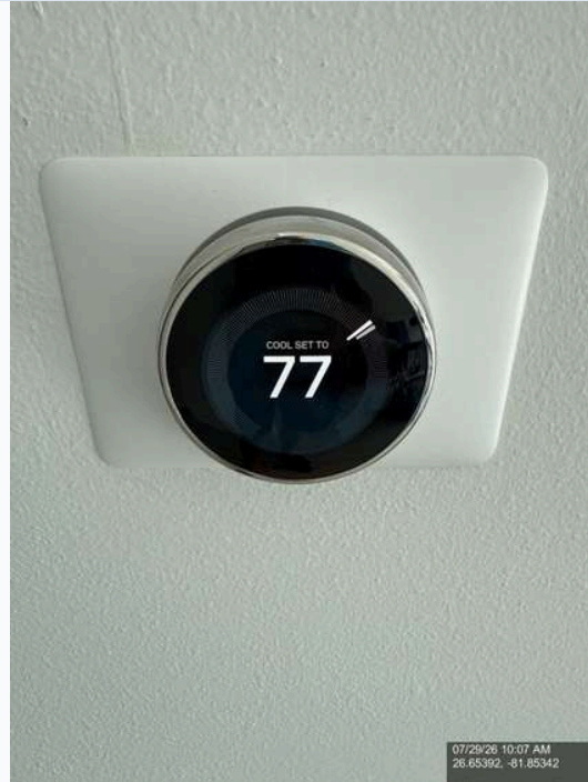
Photo 2 - Mechanical & Systems - Check thermostat for proper settings and operation
