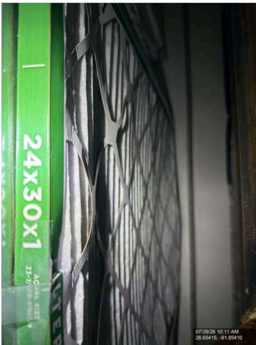
Photo 5 - Mechanical & Systems - HVAC - Filter
