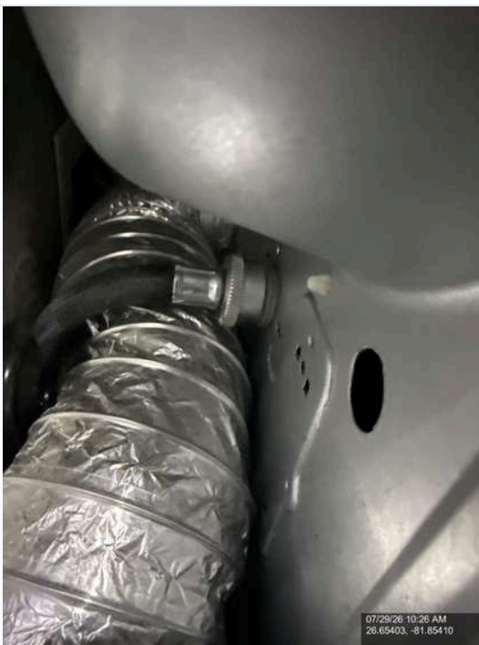
Photo 19 - Kitchen & Laundry - Washer supply hoses and dryer vent connection
