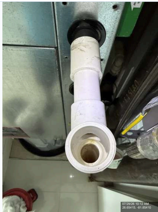
Photo 6 - Mechanical & Systems - HVAC - Drain
