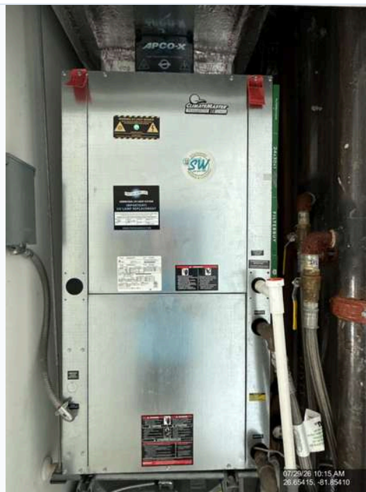
Photo 8 - Mechanical & Systems - Air handler drip pan and condensate line
