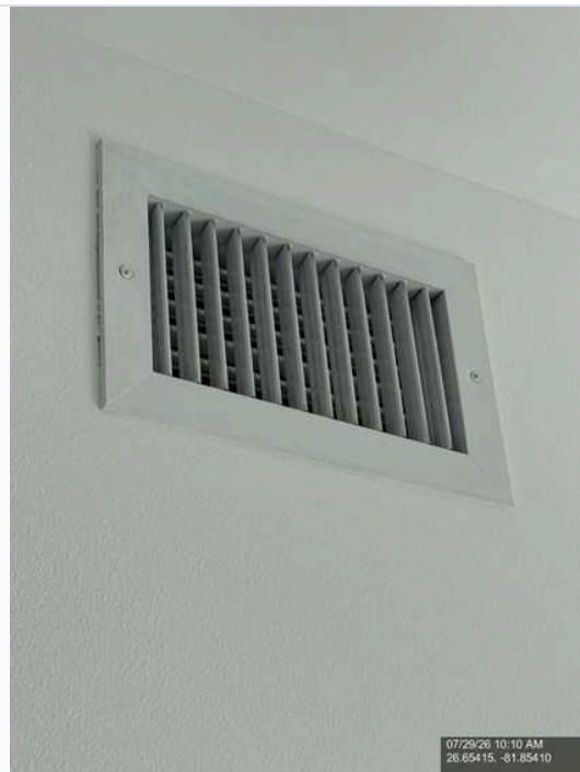
Photo 4 - Mechanical & Systems - Air handler discharge temperature at the supply vent (target 58-68F)
