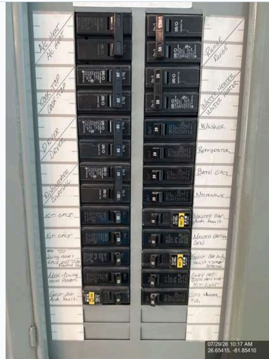
Photo 10 - Mechanical & Systems - Electrical panel: breakers set, none tripped
