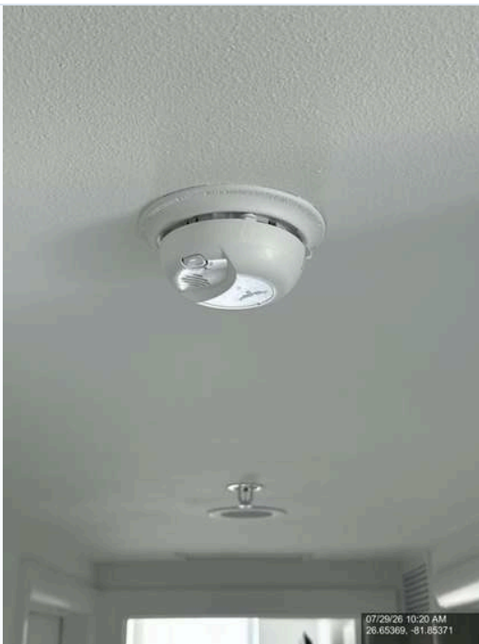
Photo 13 - Mechanical & Systems - Smoke and carbon monoxide detectors
