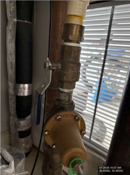
Photo 1 - Mechanical & Systems - Water main opened for this visit
