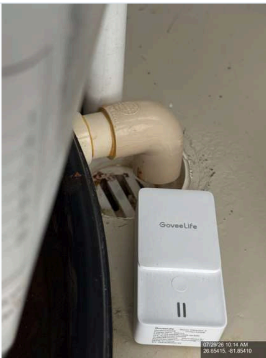
Photo 7 - Mechanical & Systems - HVAC - Drain
